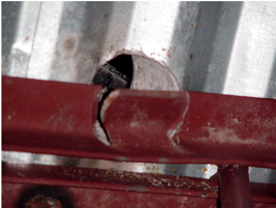
Figure 1.1 Joist Top Chord Damaged During Construction
