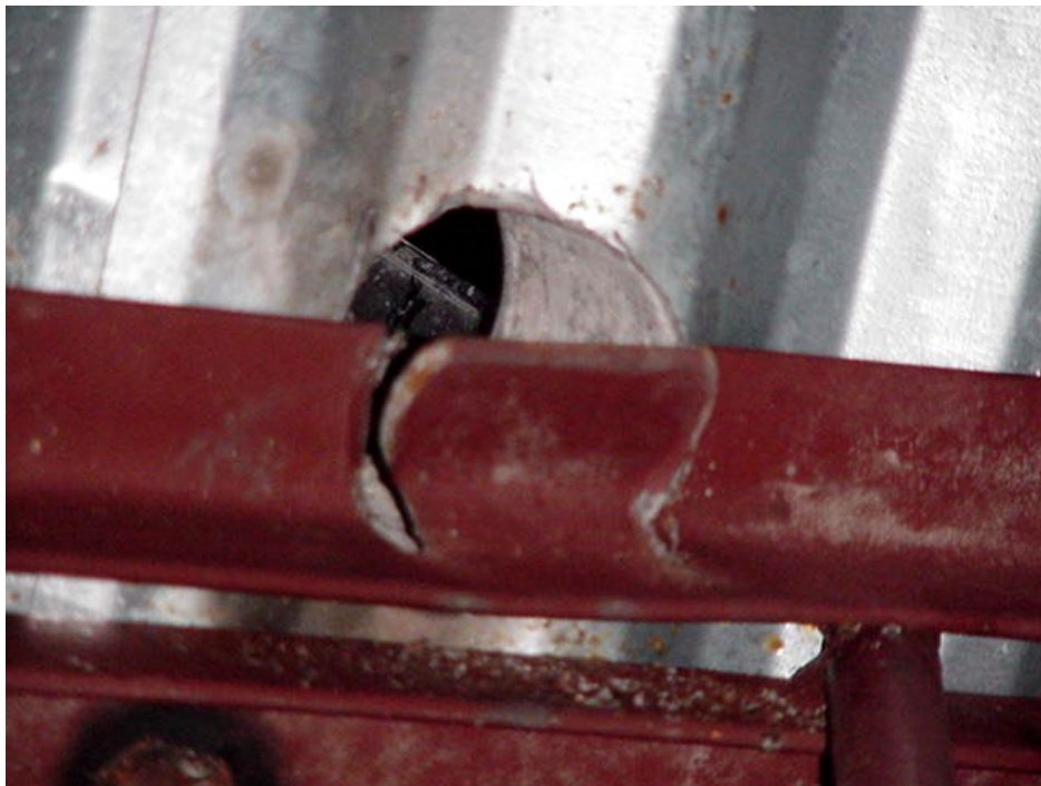
Figure 1.1 Joist Top Chord Damaged During Construction
